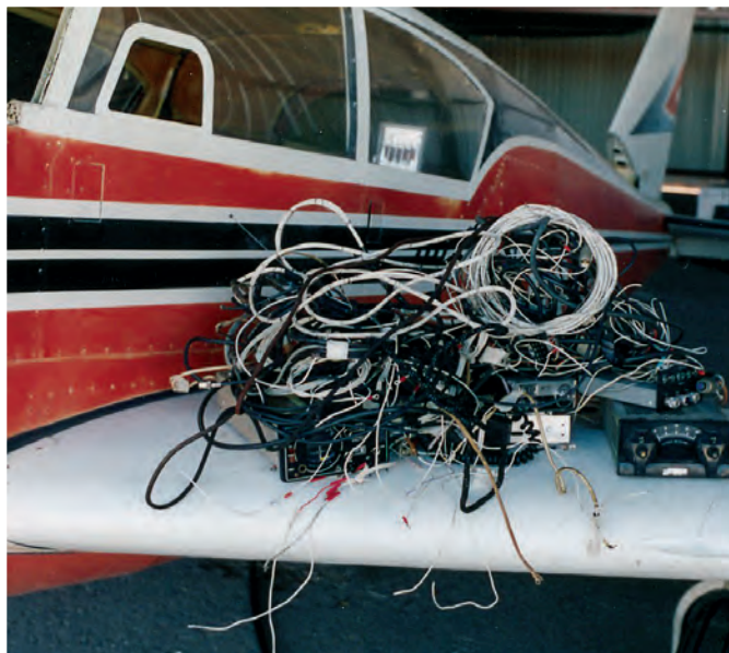
Most, but not all, of the wires removed. All of these wires must have been important in the past history of the airplane, but now had no function.
