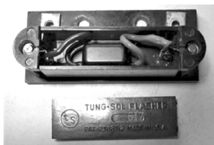
Figure 6: The repair completed with the solid-state flasher circuit inside the original flasher housing lid.
